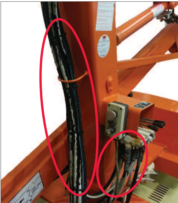
Damage along almost the full length of each hose assembly
